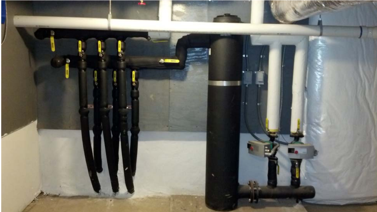
Geothermal Heat Pump System
