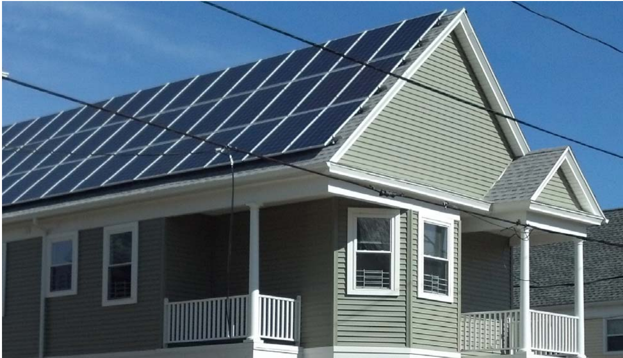
1418 West Street – PV Solar Panels
